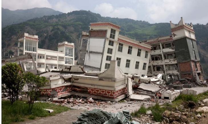
Heavily damaged school in Yingxiu, Sichuan, China, where 77 percent of the population of Yingxiu was believed to be killed by an earthquake that hit the province of Sichuan on May 12, 2008, causing 68,858 deaths.
